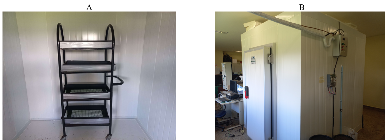
FIGURE 1. (A) Cold storage trolley loaded with trays; (B) Cold room installation.
